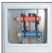
Heating Circuit Distributor
