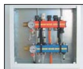
Heating circuit distributor
